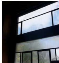
BEL Replace fogged window panes
